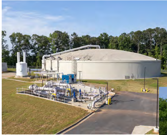
Water Treatment Facility
